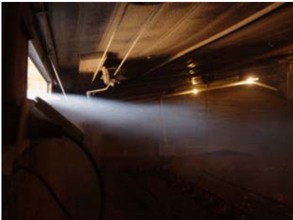
Figure 7. Air entering through wide open inlet without a light hood.
