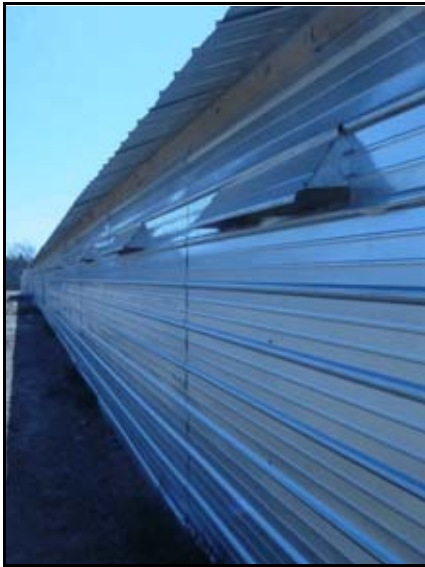
Figure 4. House with poor light hoods
