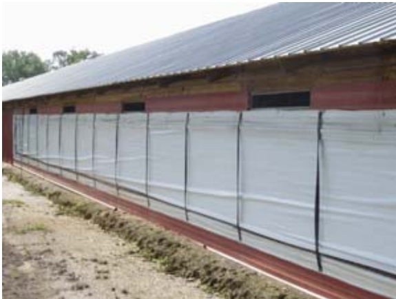
Figure 1. Side wall inlets without light hoods
