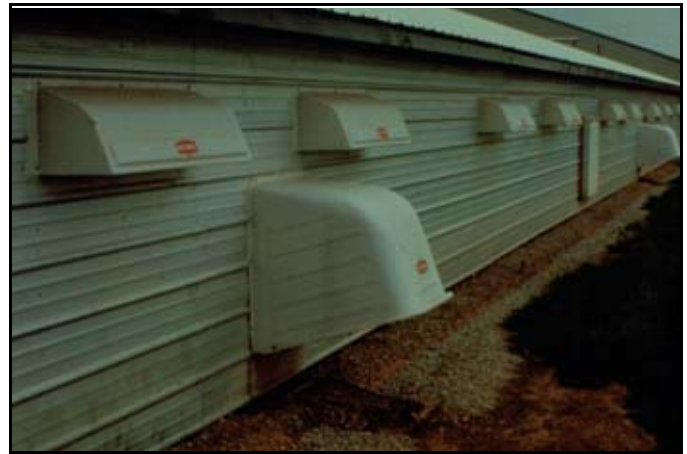
Figure 8. Large inlet and fan light hoods
